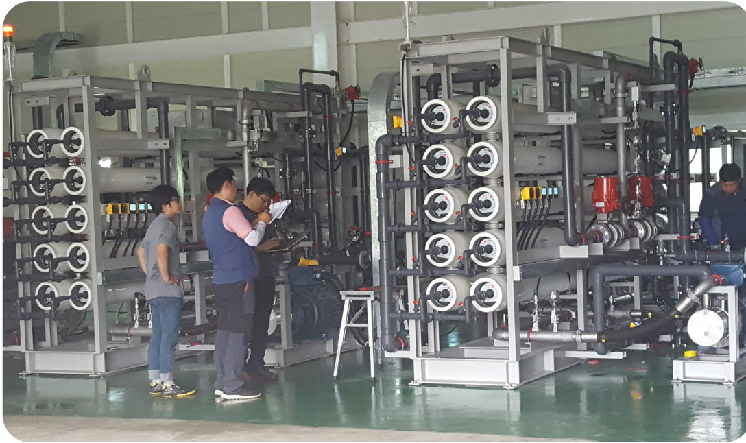
↑ The two-train, 500 CMD plant – designed around two APP 26 high pressure pumps and two iSave 21 ERDs – ensures long service intervals and built-in redundancy.
